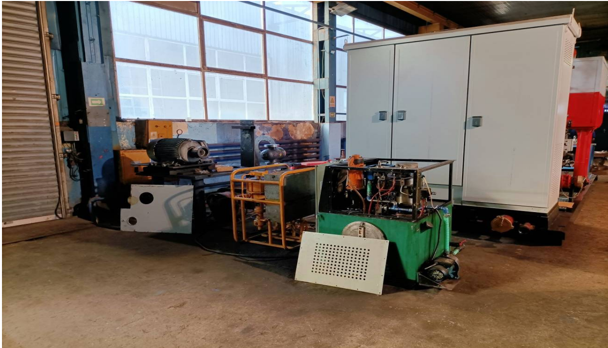
Fig 2.1- Standuri testare Instalatie de cimentare in zona dulapuri electrice
